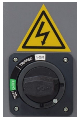
Figure 6-2: Main Power Switch
