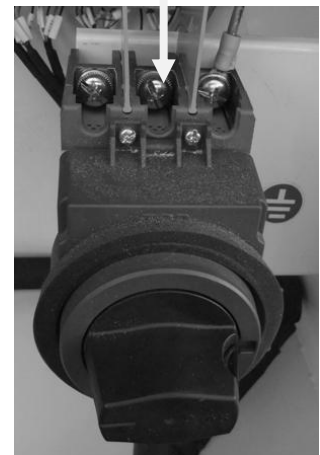
Main power switch
