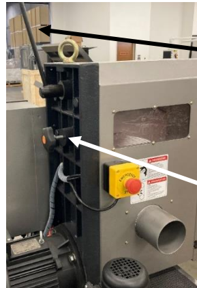
View from conveyor out-feed side (back)
