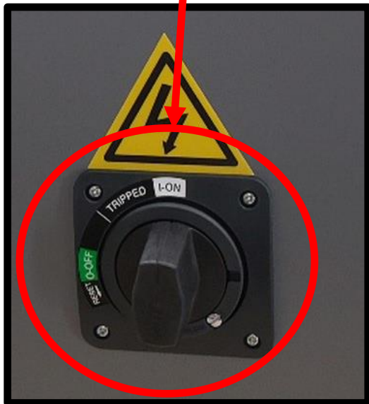
Main Power Isolation Switch
