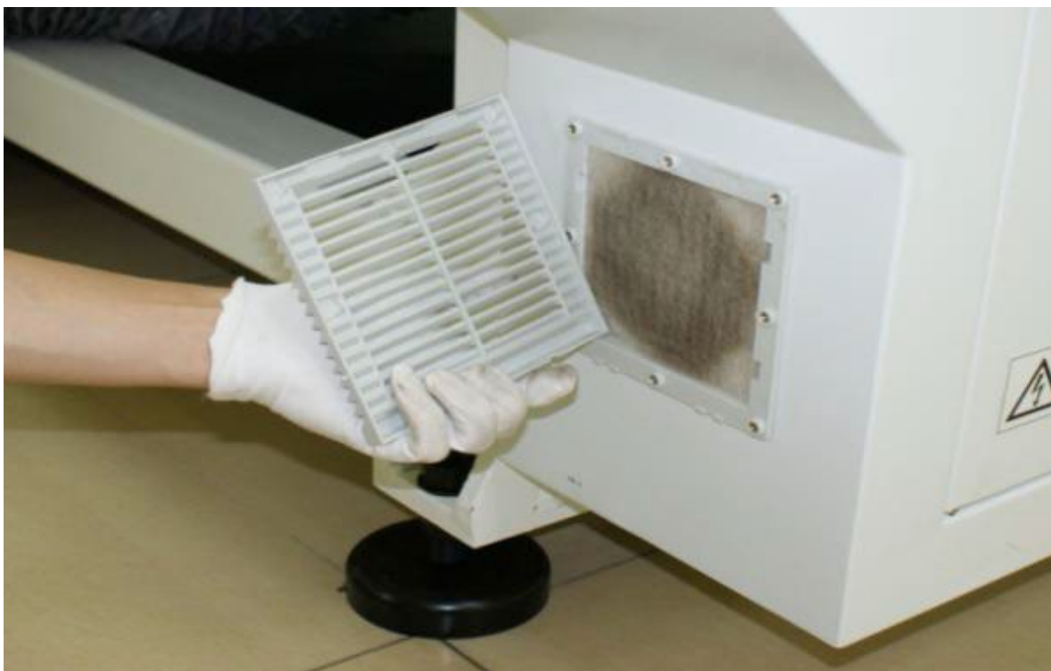
Figure 9-4: Electrical Cabinet Filter
