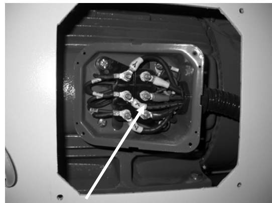
Motor electrical terminations (cover plate removed)
