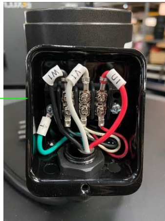
Figure 16: 110V Wiring, Junction Box
