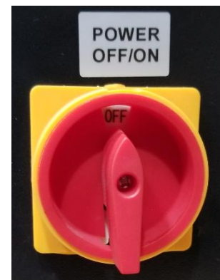
Figure 5-2: Rotary Power Switch
