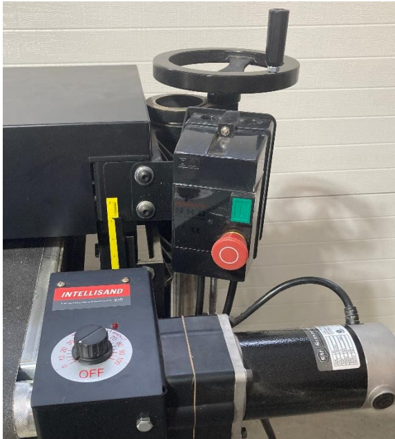
Fig. 31. Conveyor control box and on/off switch.
