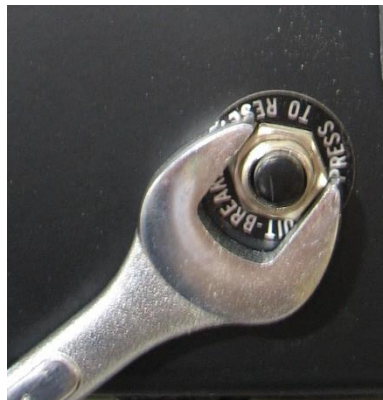
Figure 2J: Replacing circuit protector
