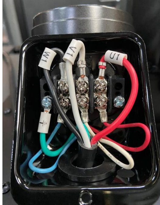
Figure 2X: 220V top wiring in auto clean junction box
