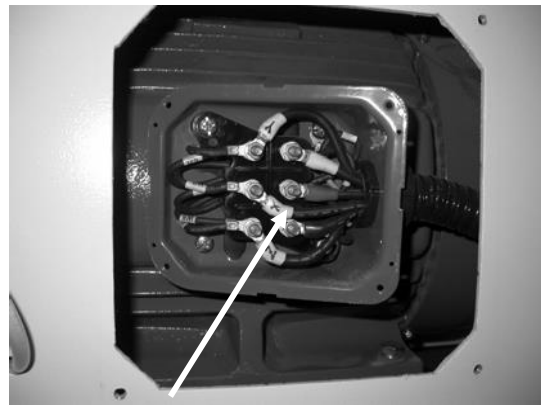
Motor electrical terminations (cover plate removed)
