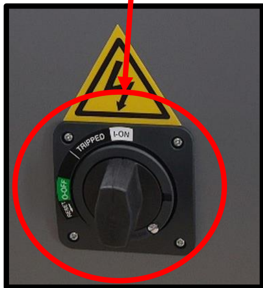
Main Power Isolation Switch
